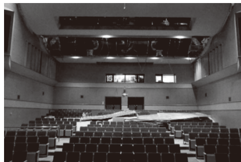
Fig. 2 Ceiling collapse occurred during 2016 Kumamoto Earthquake 2)
