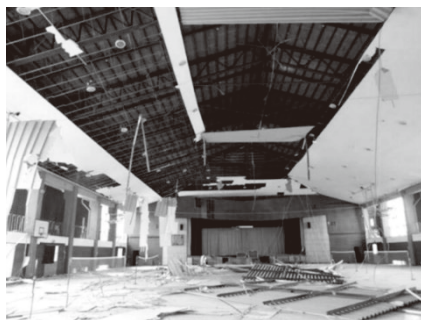
Fig. 1 Ceiling collapse occurred during 2011 Great East Japan Earthquake 1)
