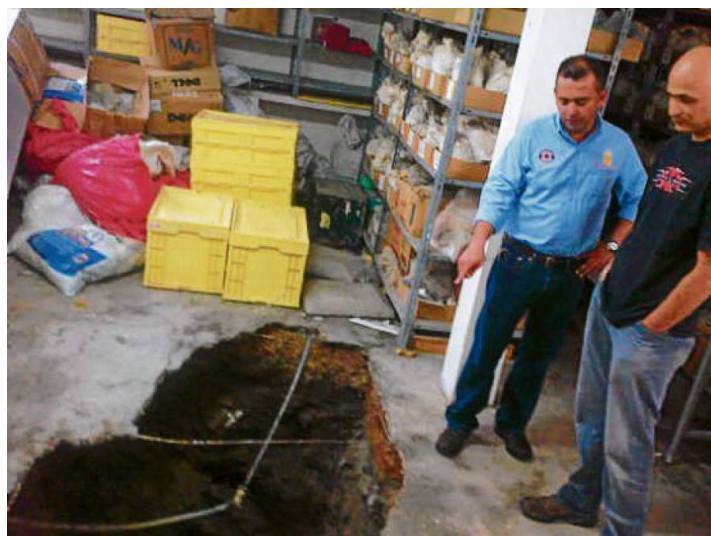
Figure 25: Hole created by a crack in the IHAH offices, source: “Ordenan desalojo del IHAH por derrumbe,” El Heraldo , http://www.elheraldo.hn/metro/709558-213/ordenan-desalojo-del-ihah-por-derrumbe
