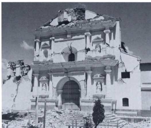
Figure 10: Cathedral with cracking above arches caused by February 4, 1976, earthquake, Tecpan, Guatemala, source: Bernard M. Feliden, Between two earthquakes (see footnote 10)
