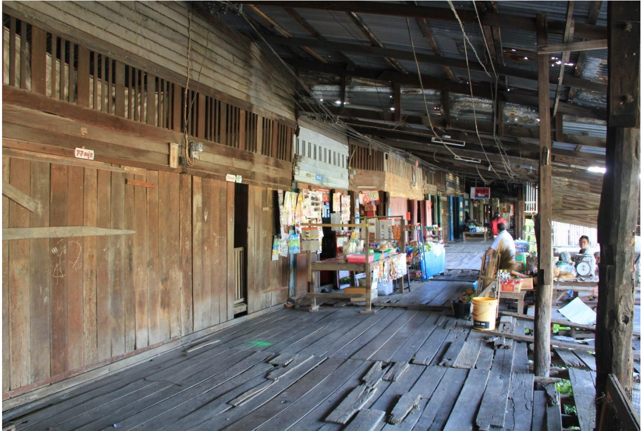
Figure 108 Abandonment in commercial community
