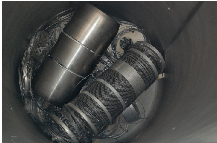
Fig.15 Photo of the fallen terminal shell and accelerator columns at the tank bottom.
