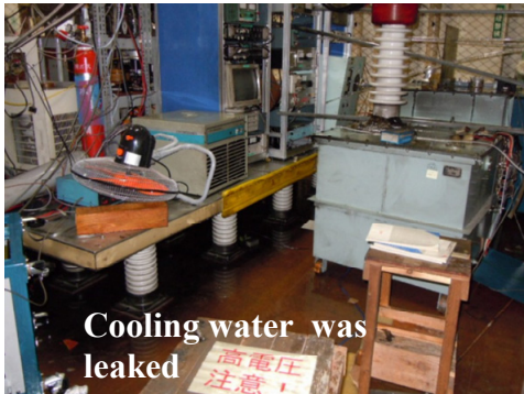
Fig.10 The flooded polarized ion source due to the broken water pressure gauges of the cooling water system.
