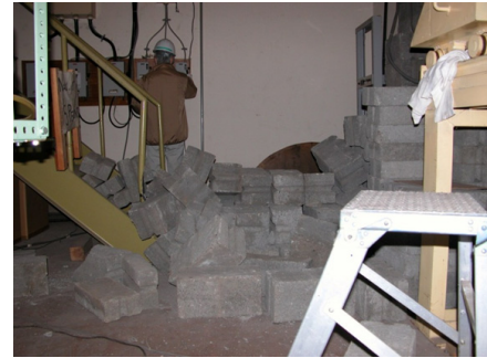
Fig.18 Fallen shielding concrete blocks at the analyzer magnet room.
