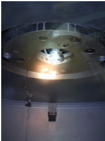
Fig.14 Lost columns inside of the tank observed from a manhole at 7th floor.
