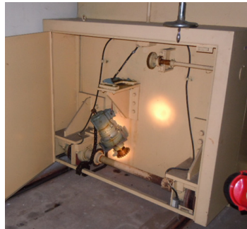
Fig.17 Broken shielding door motor at the analyzer magnet room.
