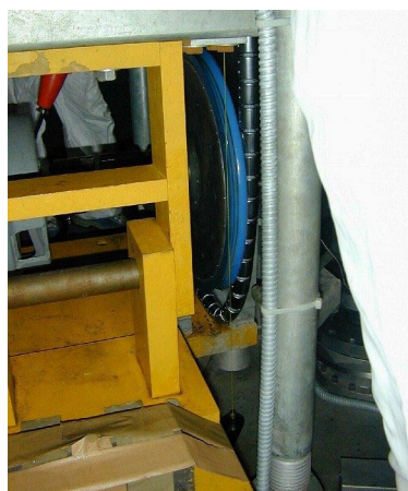
Fig.6 A plumb was hung down from the upper chain sheave to the bottom of the tank. The position of the lower sheave was adjusted with respect to the position of the plumb.
