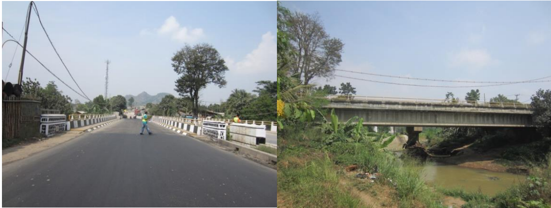
Figure B.2 Front view of Cilalawi-A Bridge Figure B.3 Long view of Cilalawi-A Bridge
