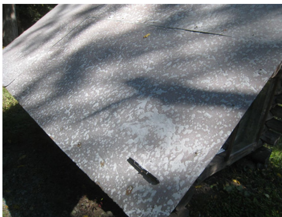
Fig. 2 Photograph of the sampling point of pyroclastic material OT-1, the roof of a garden shed at the Kanose hot spring, in the morning of September 30, 2014
