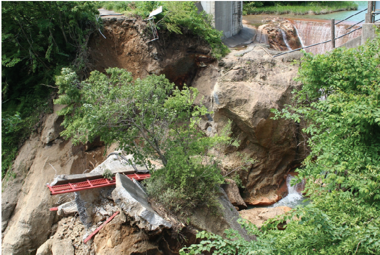
Fig. 23. Collapsed footbridge downstream (length is 24 m) at Yabitsu Dam / Weir site.
