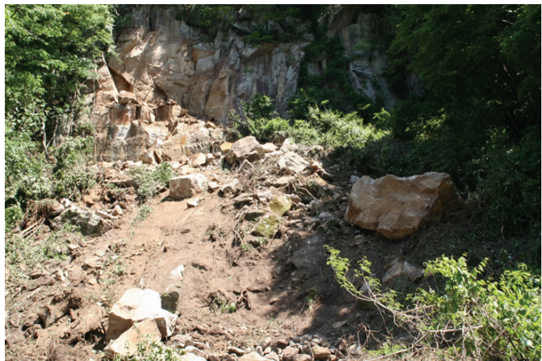
Fig. 20. Close-up of Ichinoseki Genbi-Itagawa small-scale slope collapses near National Route 342.
