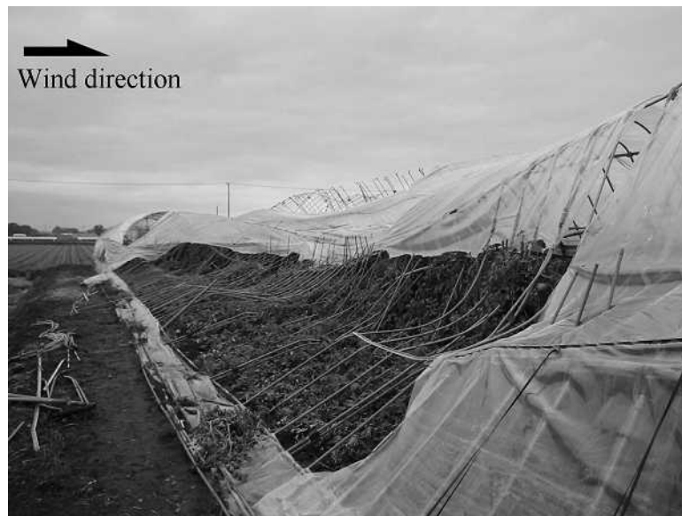
Fig. 2.12 Mode of collapse for pipe house constructed in open and flat ground: the pipe house showed was pipe house A.
