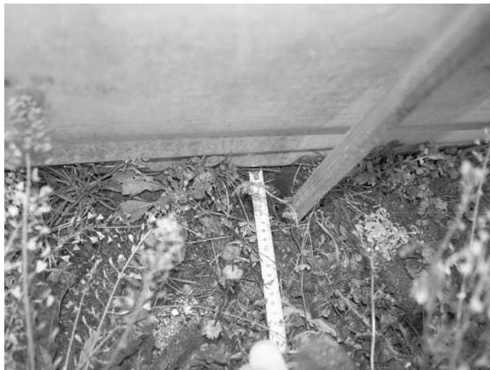
Fig. 2.8 Horizontal displacement of arch pipe at the ground level.
