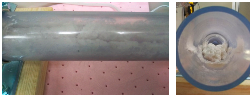
Figure 4. Clogging inside the sewer pipe on the 7th day in the simulated experiment (Observation point 4).
