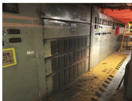
Switchgear Room after the event
