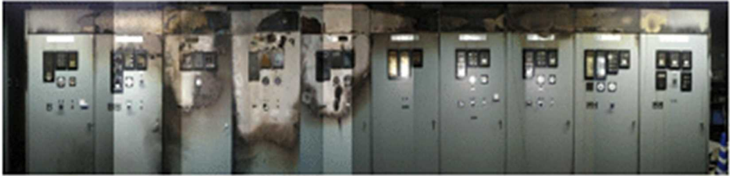
Fig. 2.2—7 Ten connected cabinets with damage after the fire [11]
