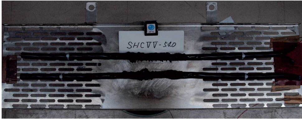
SHCVV cable temperature 340°C
