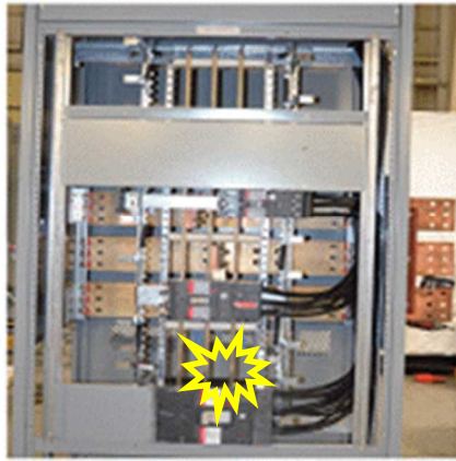
Arc point at the rear of DP
