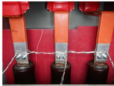
(b) Short wiring for Arc
