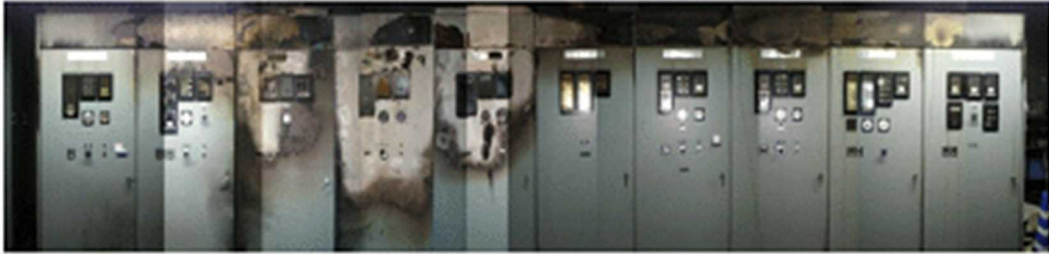
Fig. 2.4-4 Ten connected cabinets with damage after the event [11]
