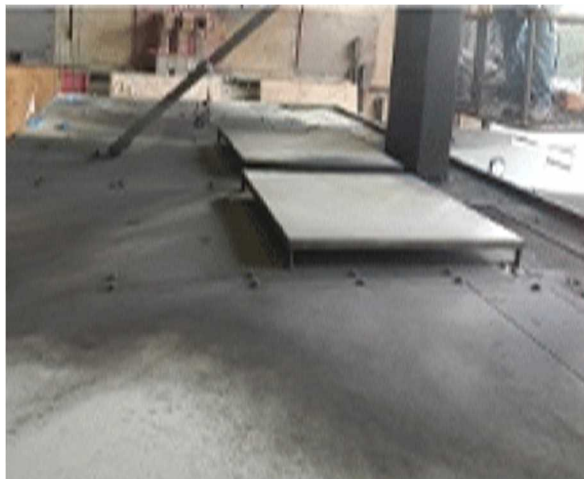
Fig. 2.5—13 Top of cabinets after SWGR Test 1 The top of the cabinets had some soot deposits and minor scorching where the arc discharged through the top vent. [12]
