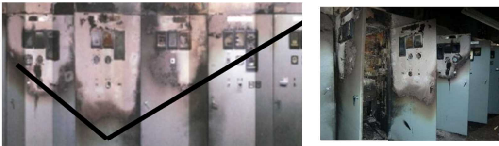
Onagawa post-fire damage
