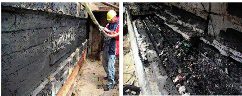
Fig. 2.2-3 Photos of cable damage;
