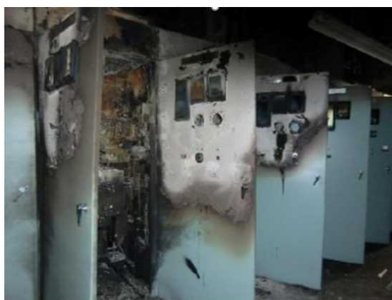
Fig. 2.2-6 Electric cabinet with the sector on the left where the fire started [1]
