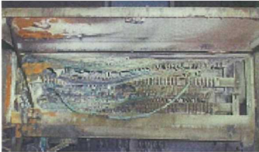
Fig. 2.2—8 Damage after the event in the control duct [11]
