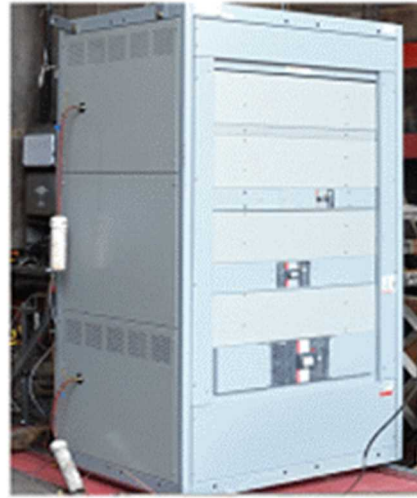
Exterior of DP
