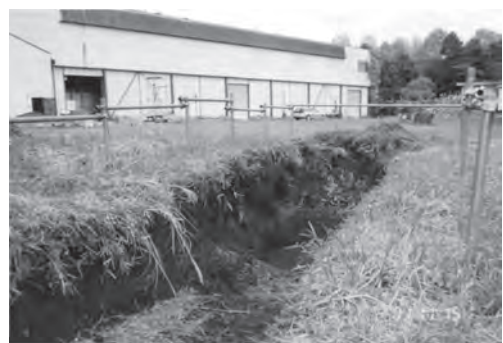
Photo 1 Condition at the trench
